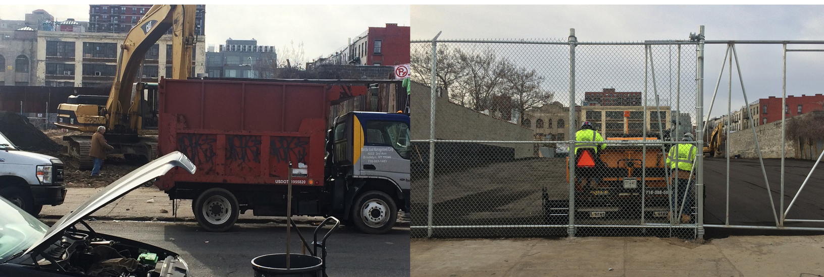
IMAGE: THE WEEDY GROUND ACROSS FROM THE EPA ENTRANCE GETS LEVELED AND SURFACED WITH ASPHALT
